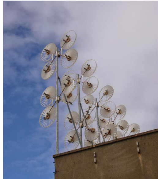
Micro Wind Generation Turbines on site © Gäbler 2013
